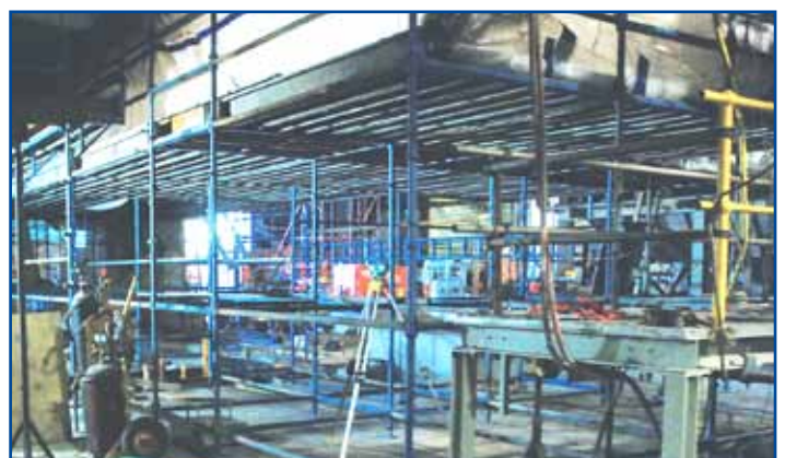
Foundation work on the Unit 6 Ash Hopper is being carried out by Walz Construction.
