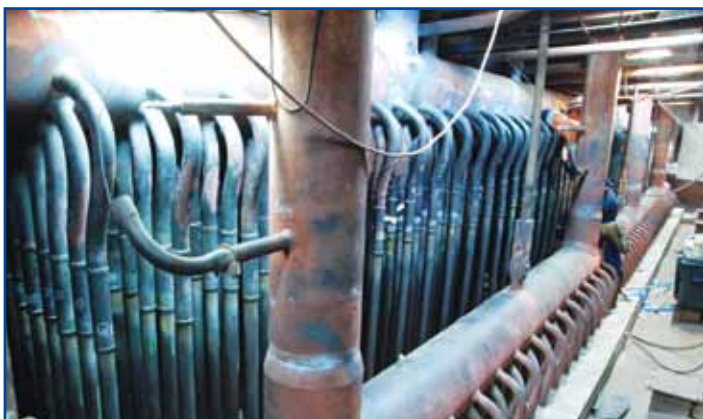
Replacement of the welds of the dissimilar metals is being undertaken in the boiler penthouse.
