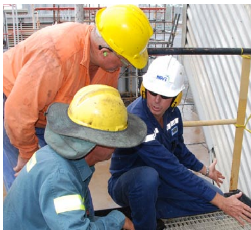
Rick Thomason discusses the handrail project with Walz Construction employees Darren McNeil and Noel Christensen.
