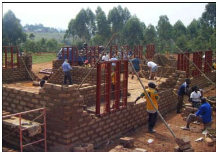
The teams get to work building the new homes for the homeless children
