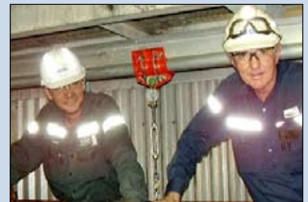
Ashley and John were happy to pose for a photograph after installing a new monorail on Unit 4 boiler.
