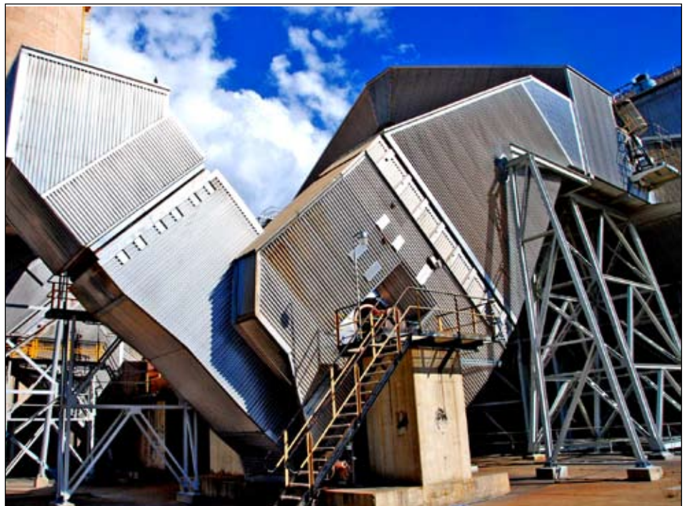
Work is currently underway on reducing the noise levels around the Induced Draft Fans at the station
