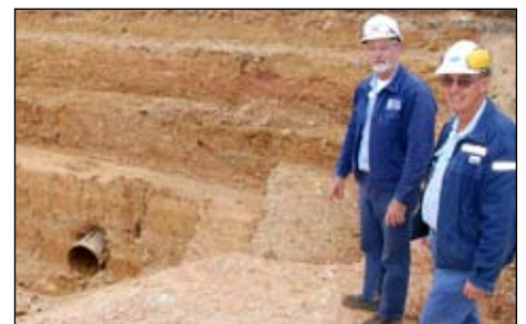
Graham Long and Allan Timm inspect the new cable route being constructed near 1-4 CW pumps.
