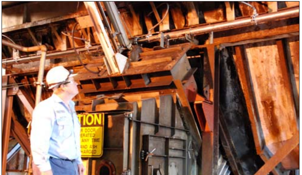
Kevin Creagh inspects the ash hopper on Unit 1 which will be refurbished in the next few years.
