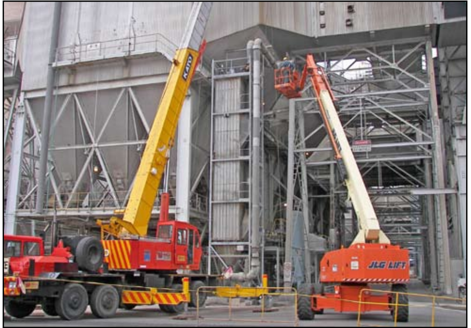
The fabric filter pilot plant was recently demolished as part of the hazard reduction program.
