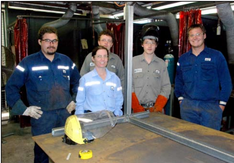
NRG's Michael Zimmerlie, Kate Williams and Luke Halliwell assist GSESC students Sam Carter and Josh Little with the construction of a portable welding station.
