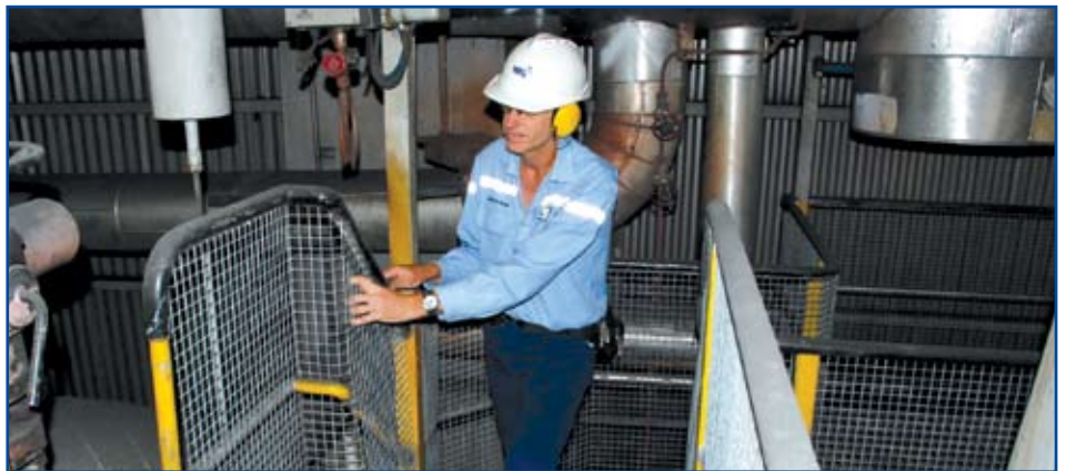
Dave Greinke inspects some of the mesh that has been installed around the boiler handrails.
