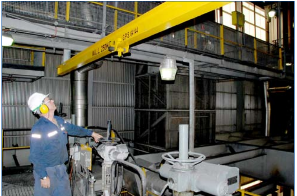
Kev Johnson checks out the monorail beam which has reduced the potential for injuries for employees carrying out maintenance on the valves.
