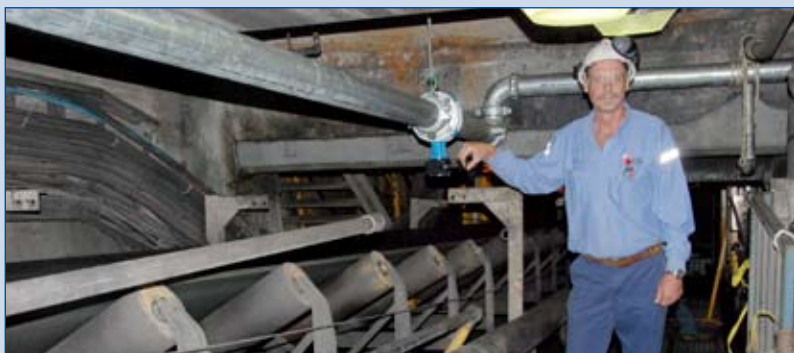
Fairbairn Engineering Services Project Manager Gordon Low is managing the refurbishment of the coal unloading track hopper building.
