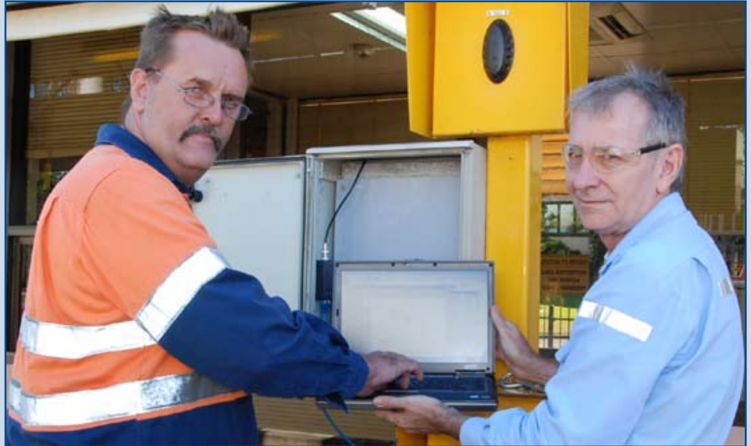
John Illingsworth and ADT Security technician, Gregory Mollenhauer fine tune the new I Track system.
