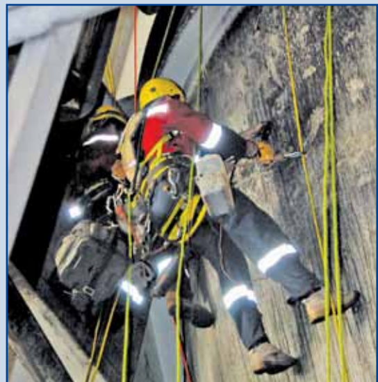
Highpoint Access and Rescue staff carry out thickness measurements on the outside of the bunkers.
