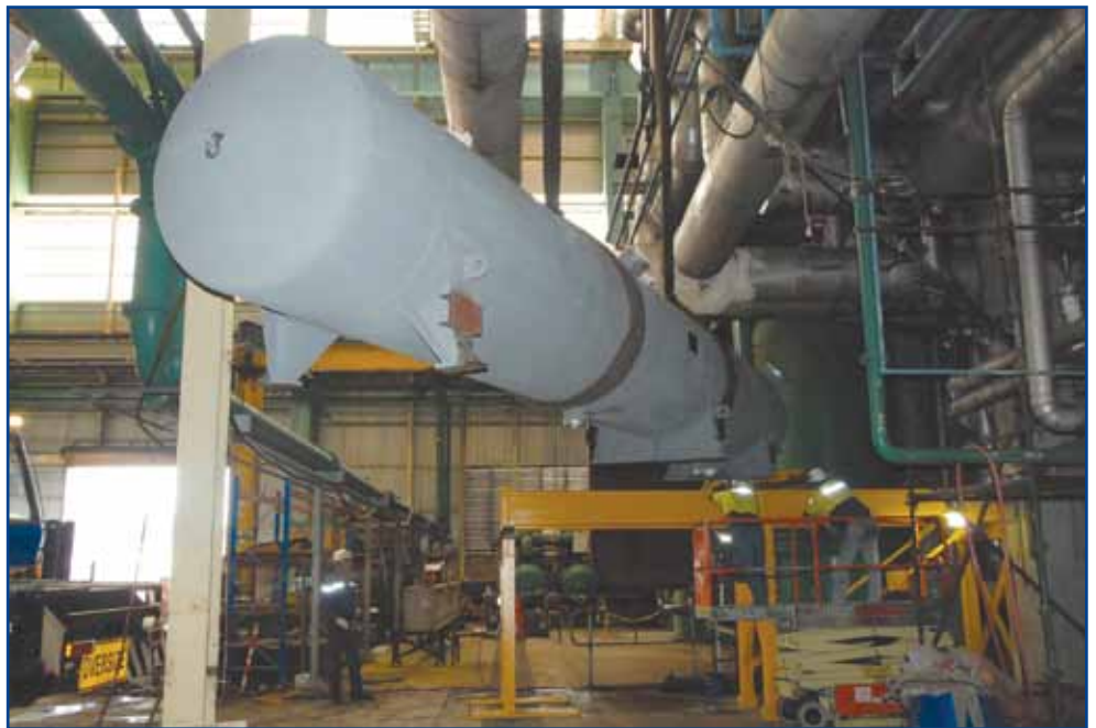
This is the first time LP heater 1 had been replaced since the station was originally built.
