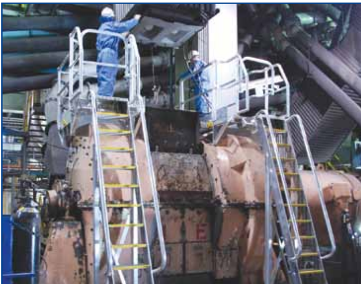
Gavin Donohoe and Bob Watts test the new platforms which have improved safety around the pulverisers.
