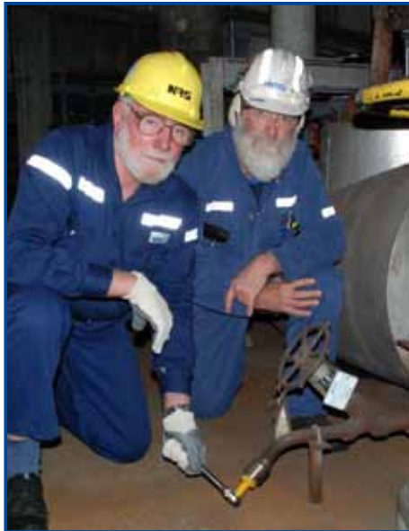
Greg Nugent and Michael Jess inspect the newly modified drain plugs in the feed heating area.
