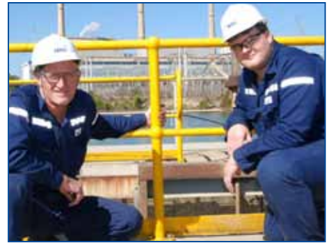
John Hall and Brad Zillman fabricated the new handrails around the 1-4 detention ponds.
