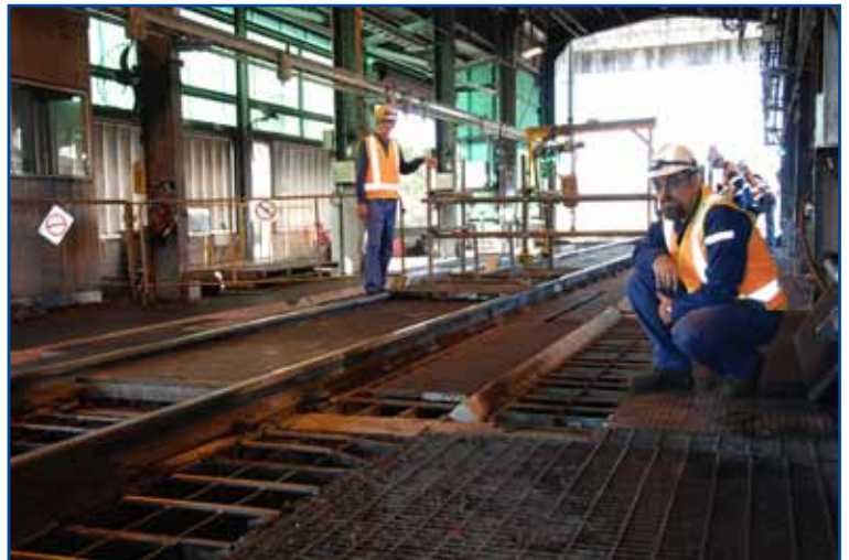
Larry Brushe and Mark Fleming inspect the widening of the unloading grizzly bars as part of the refurbishment.
