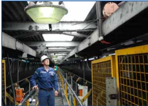
Fuel Superintendent Matt Adamson checks out the improved visibility between T3 and T4 transfer towers.
