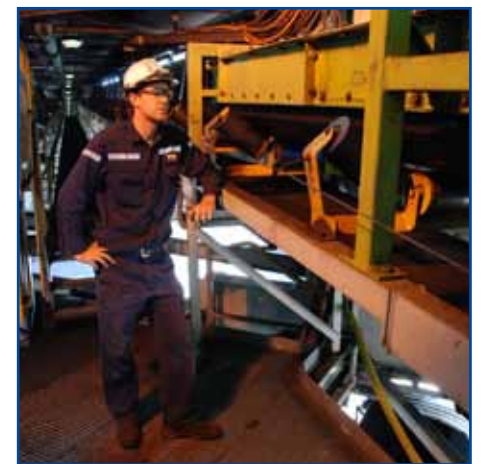
Craig McGuinness came up with the plan to extend the coal chute around c34 coal chute
