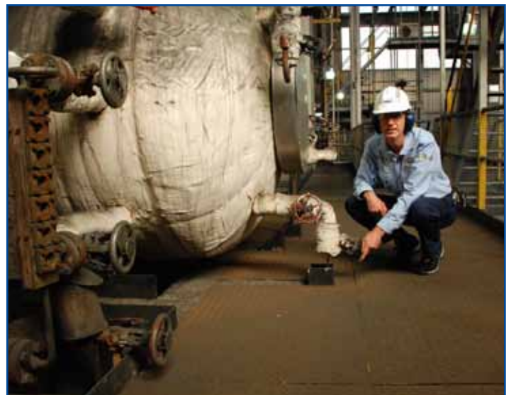
Dave Greinke checks out the checker plate that has recently been installed around the boiler drums on each unit.
