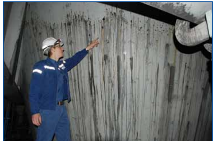
Ross McKenzie inspects the corrosion on the coal bunkers.
