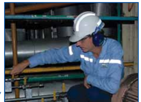
The new ball valves are now more accessible.
