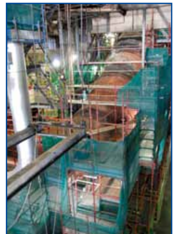
The photo shows the replacement of the cladding and insulation of the Unit 2 flue gas duct.
