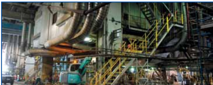
Civil works is being undertaken in preparation for the new ash hopper.
