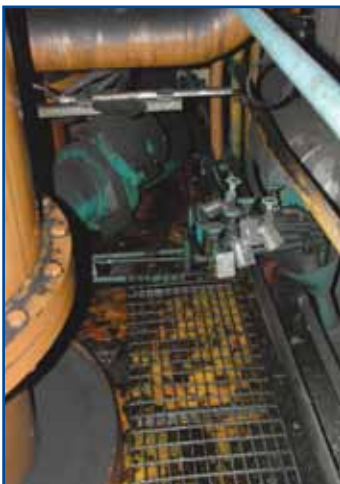
Isolation Officers had difficulty accessing the old valves.
