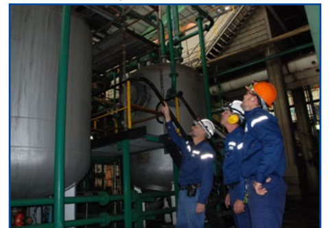
Mick, Bob and Grant inspect the work recently carried out on the Z Polisher Systems.
