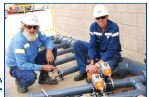
Rob Brown and Rick Thomason inspect the hypochlorite pipework.
