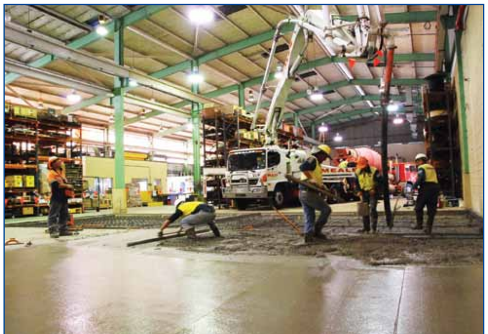
Oaka Engineering employees repair the concrete slab that was damaged following a pipe rupture last month.
