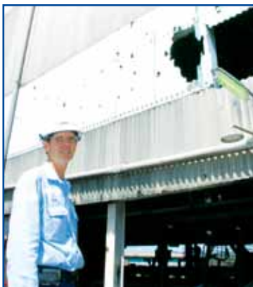
Dave Greinke checks out the wall sheeting that is being replaced as part of this year's hazard reduction.
