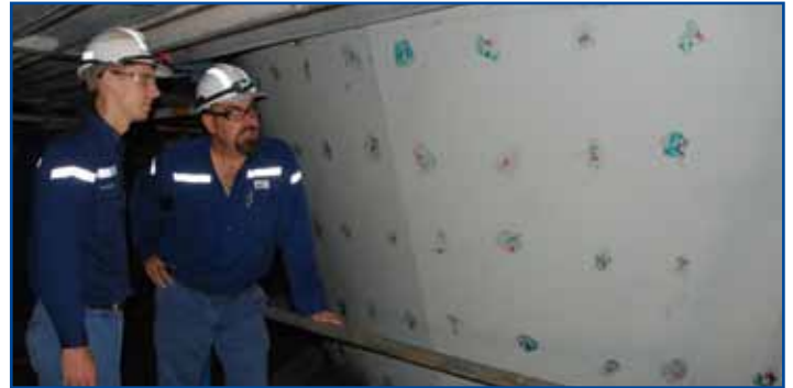
Ross McKenzie and Mark Fleming check out the work to be done on Unit 3 coal bunker.
