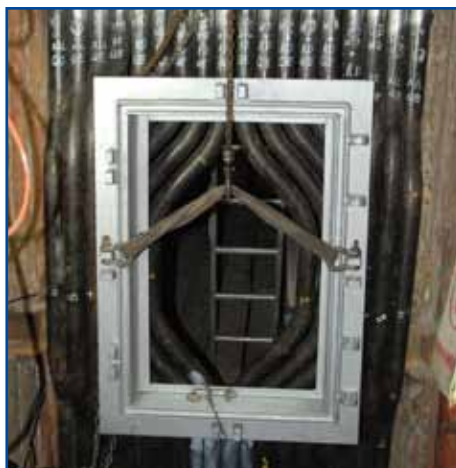
The new boiler access door.
