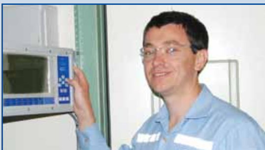
Glen inspects the upgrade to Unit 3 Turbine and Feed Pump Vibration System.
