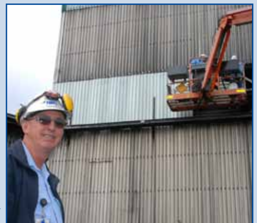
Allan Timm checks out the repair work being done on the transfer towers.
